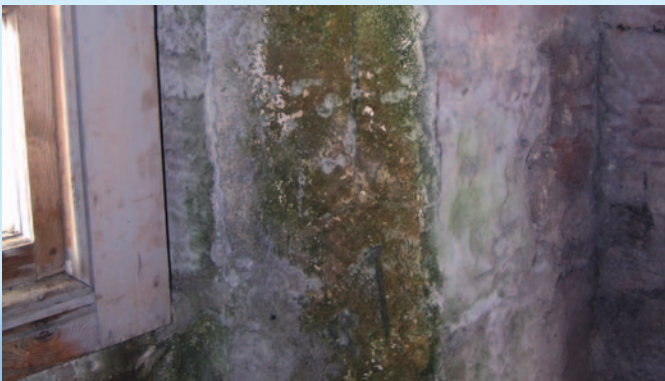
Inside test area, showing salt damage at Blickling
