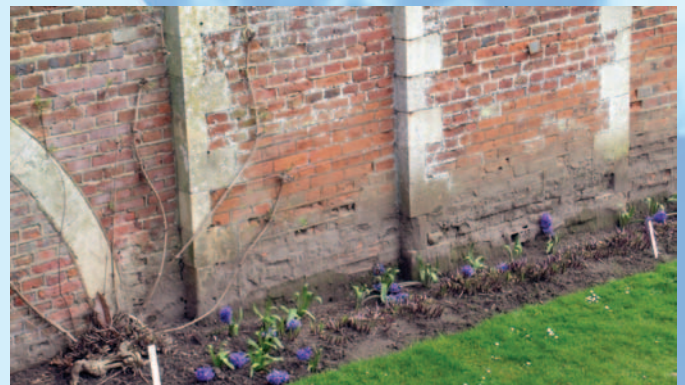
Exterior of test area, showing brick damage at Blickling
